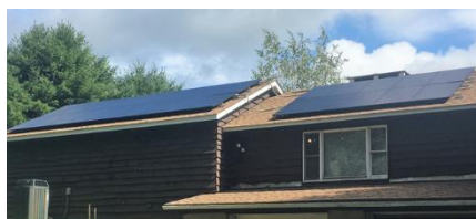
Lacawac Sanctuary's New Solar System
